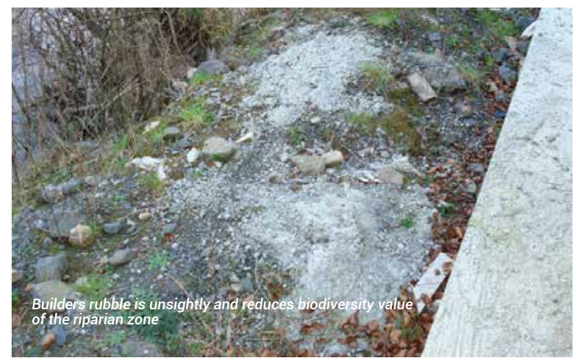
To accommodate this development the adjacent land has been raised too close to the river. This recently built retaining wall almost entirely eliminates the riparian zone and eliminates anglers access. The height of this wall has also introduced another hazard to the area, arguably more dangerous than the river itself to children and local residents.
